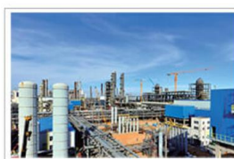
Energy and Chemical
