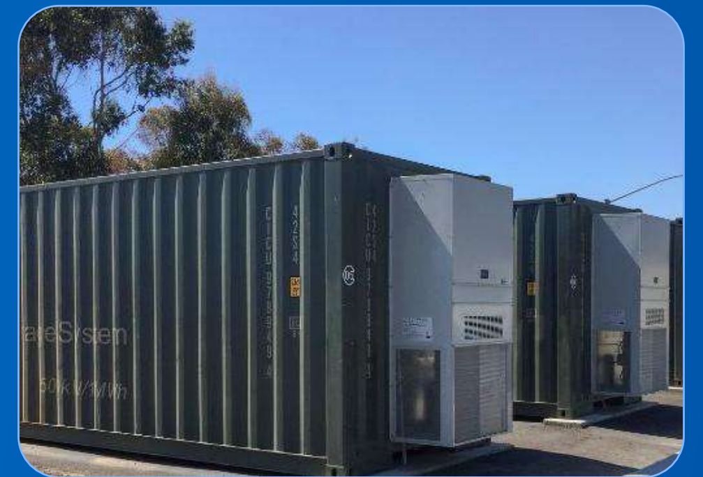
▲ EMS for Energy Storage
